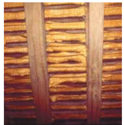
Figure 14 Sprayed foam used as a way of avoiding stripping a 'nail sick' roof and providing some insulation is NOT recommended good practice on a historic building. (Photograph courtesy of Kevin Stubbs, Bursledon Brickworks Conservation Centre)
