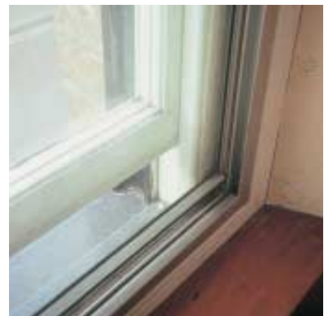
Figure 9 Secondary glazing can provide very effective thermal improvement. In historic buildings its successful insertion depends on fitting within the reveal in such a way as not to damage historic fabric. However, secondary glazing can sometimes produce an unsatisfactory reflection when viewed from the outside. (Photograph courtesy of Kit Wedd)
