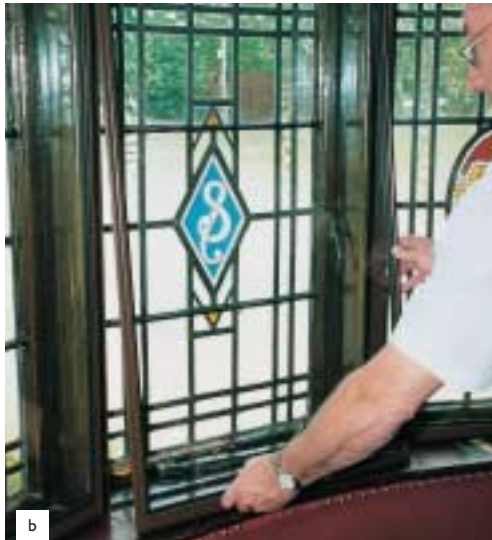
Figure 16 The heat loss from this listed public house has been dramatically reduced by the installation of discreet secondary glazing (b) and (c). The glazed panels can be easily removed in summer. (Photographs courtesy of Storm Windows, Leeds, © copyright Storm Windows, Leeds)
